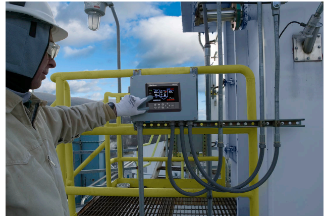
Operators access control and diagnostic functions from the B-PAC™ control units at the process, or remotely using FilterWARE™.
